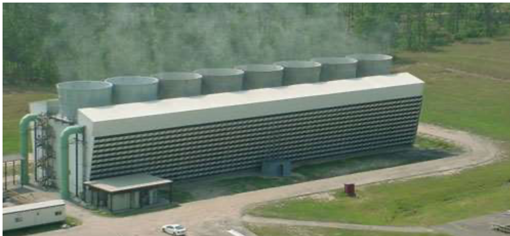
Example of 8-Cell Cooling Tower
